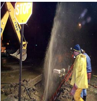
DPW attends to a Water Main Break.
